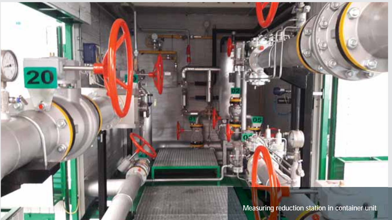
Process connection of liquid ring compressor skid unit
